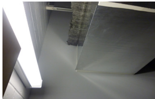
Figure 11. Air Conditioning Ducting Penetrate The Partition from The Receiver Room to The Source Room (Personal Documentation)
