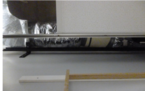
Figure 10. Air Conditioning Ducting Inside The Receiver Room (Personal Documentation)
