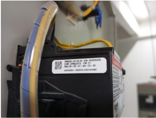
Fig. 2. MAC address on PowerLogic PM5560 installed on Chiller 2
